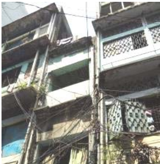
Fig. 5. Congested building space at Shakhari bazar with non-designed extensions surveyed in the research
